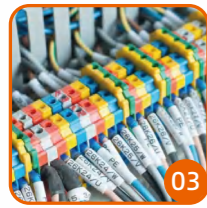
Access Control System
