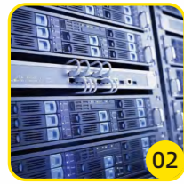
Network Cabling System
