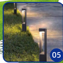
Outdoor Lighting System
