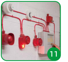
Fire Protection and Alarm System
