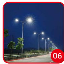
Lighting Control System
